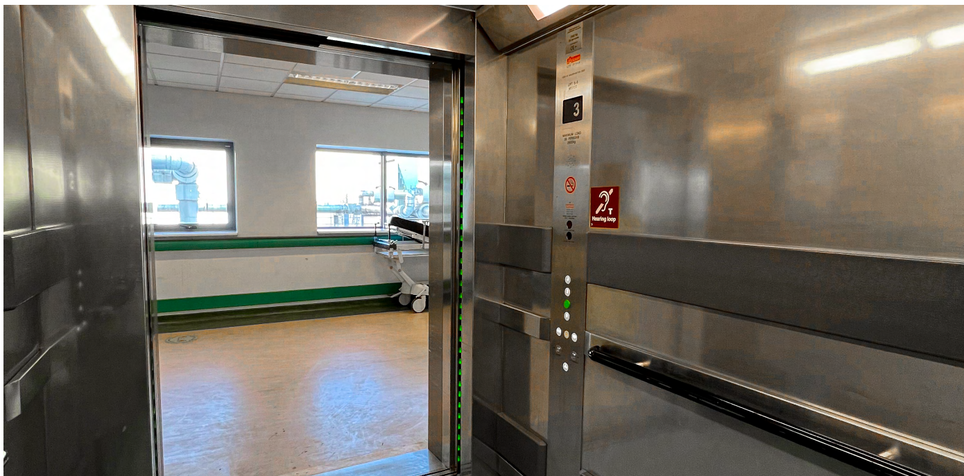
Typical hospital bed lift installed and maintained by Jackson
